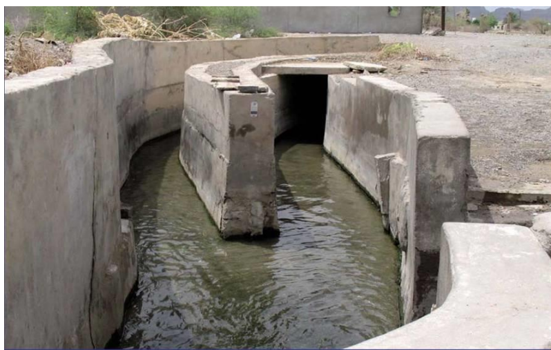
Fig. 4: High water flow with no intevension to the canal
